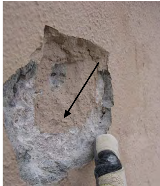
Figure 6 Test area 3, center of right side. Top layer of cement is visible, arrow indicates cut into concrete substrate
