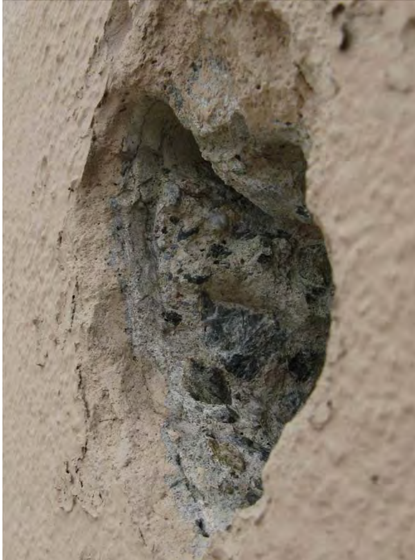
Sample 6: Core - drilled sample area showing stucco layers and concrete substrate. Dark spots are concrete aggregate
