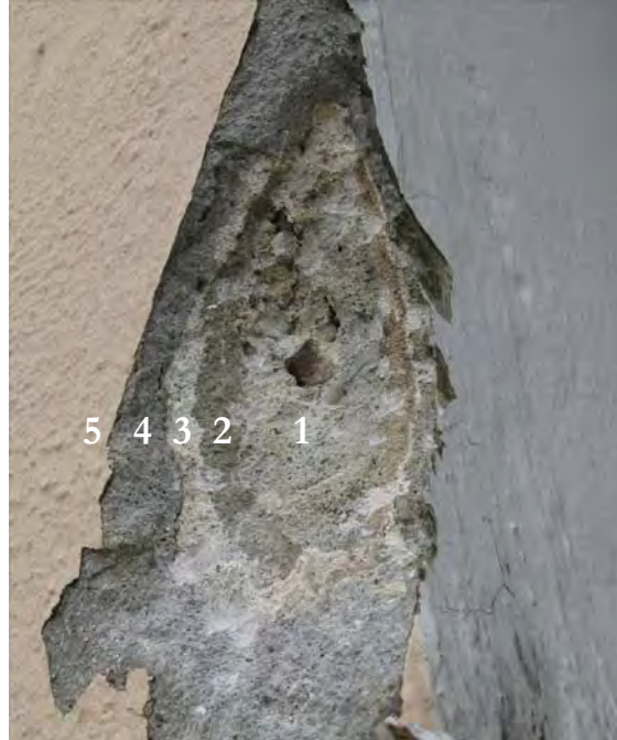
Figure 5 Test Area 5 from the corner of the arch. layers include: 1-reinforced concrete; 2-base coat; 3-lime setting bed; 4-cement stucco; 5-paint
