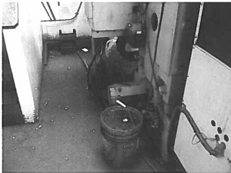
Photo 2. View of floor staining adjacent to various cutting machine inside Production Specialties (Photo date: March 29, 2013).
